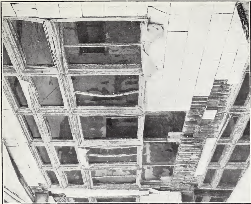
B. FAILURE OF TERRA-COTTA TILING AND METAL-FRAME WIRE-GLASS WINDOWS BY FIRE; LIGHT-WELL COLUMN, WELLS-FARGO BUILDING, SAN FRANCISCO.
